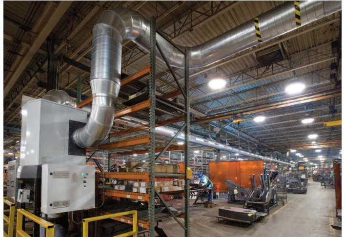
Elgin's push/pull system was installed in the high-volume chassis welding area.
